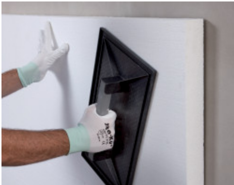
Pressing the panel in place to guarantee a good bond to the substrate
