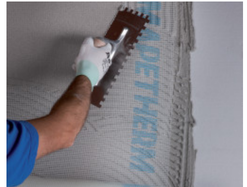
Application of a reinforced smoothing and levelling layer by embedding Mapetherm Net
