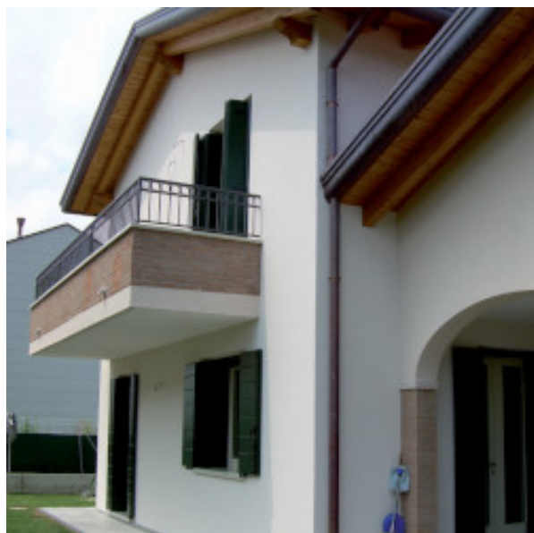
Reggio Emilia - Italy - Work on a private home using Mapetherm ARI GG
