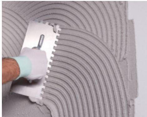
Laying of the first coating of smoothing compound with Mapetherm ARI GG
